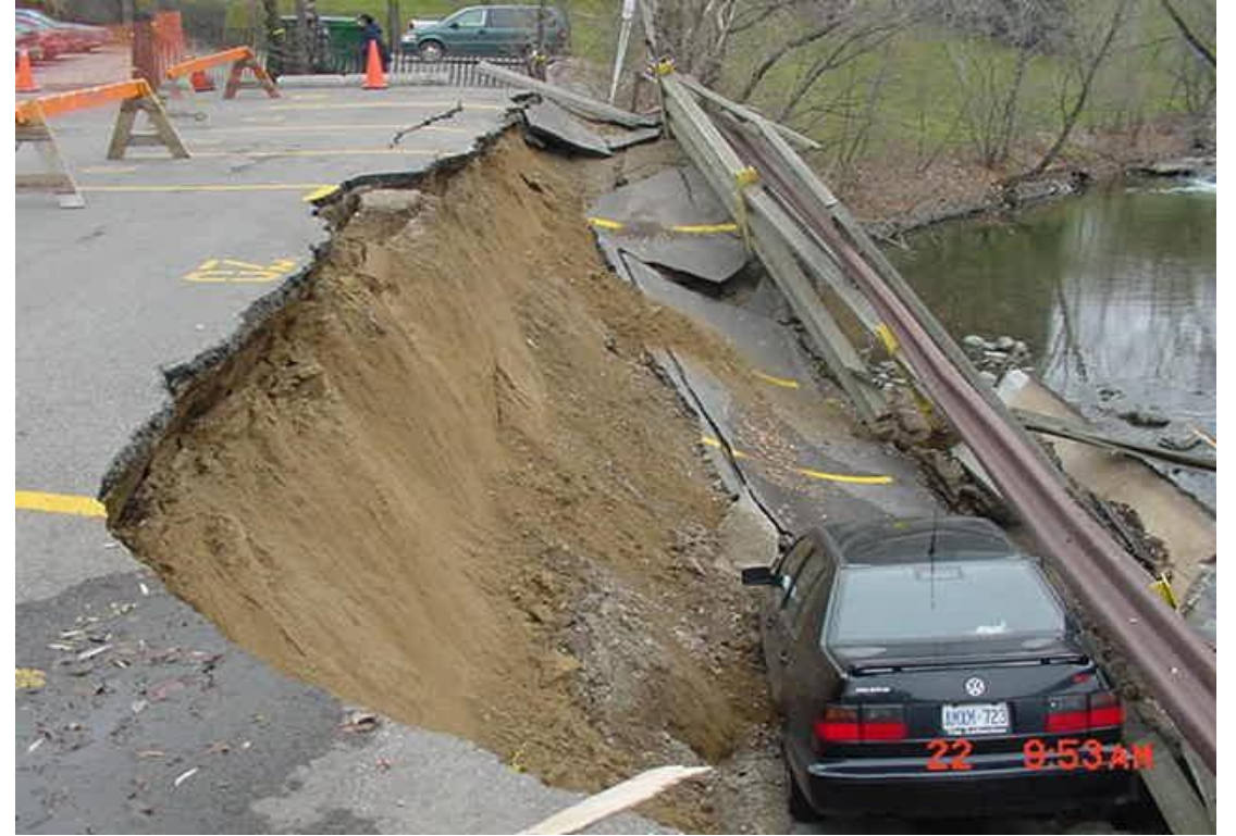
Cooksville Creek Flooding and Erosion
